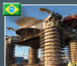
offshore platform etesco millenium
